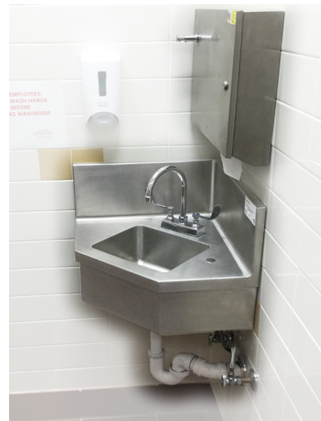
WS-CK Installation at Sampson G. Smith Middle School
